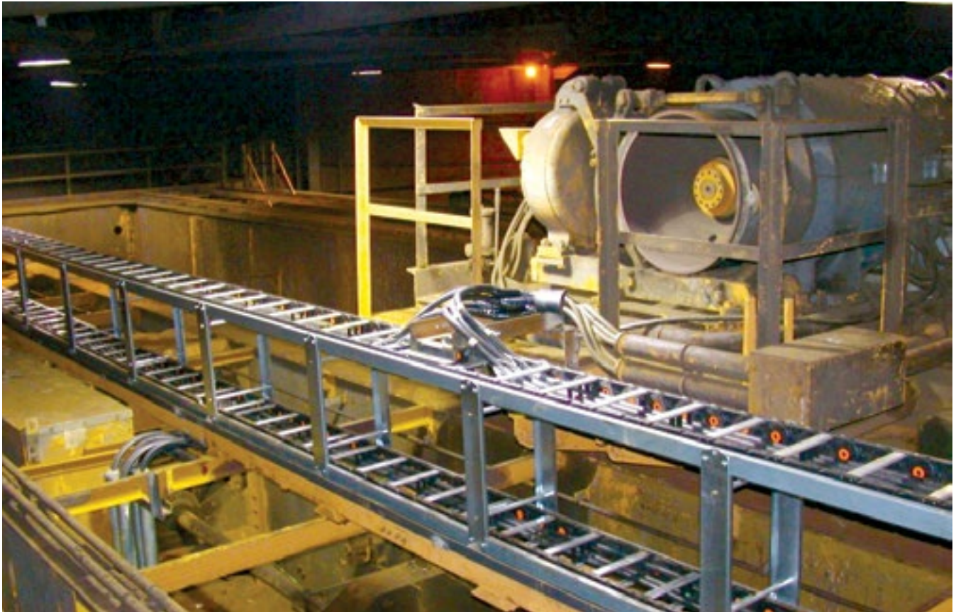
A complete cable carrier system designed by Dynatect includes a high-velocity rolling carriage and Nylatrac ® Modular TL carriers to achieve long travel in a steel mill.
